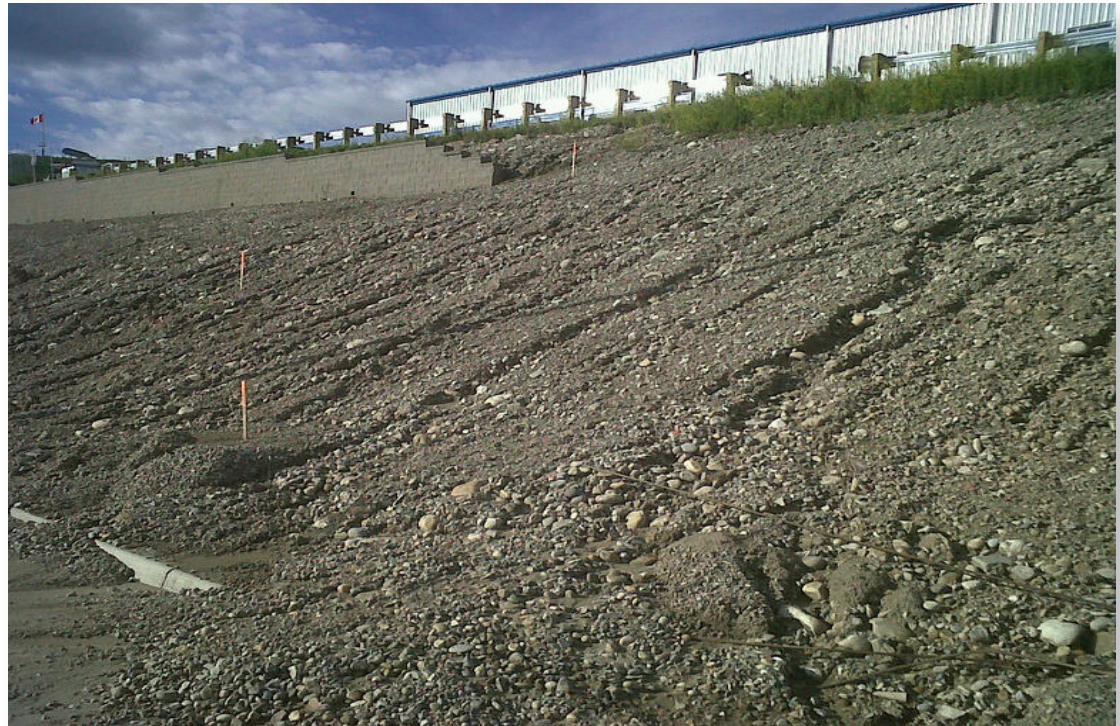
Steep, highly erodible slopes made the placement of erosion control products difficult, 2011
